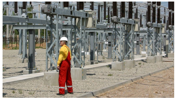
The switchyard in Alytus will be completely reconstructed
