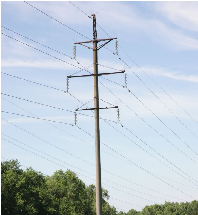
The Kretinga-Benaičiai overhead line will control current power transmission flows in Western Lithuania
